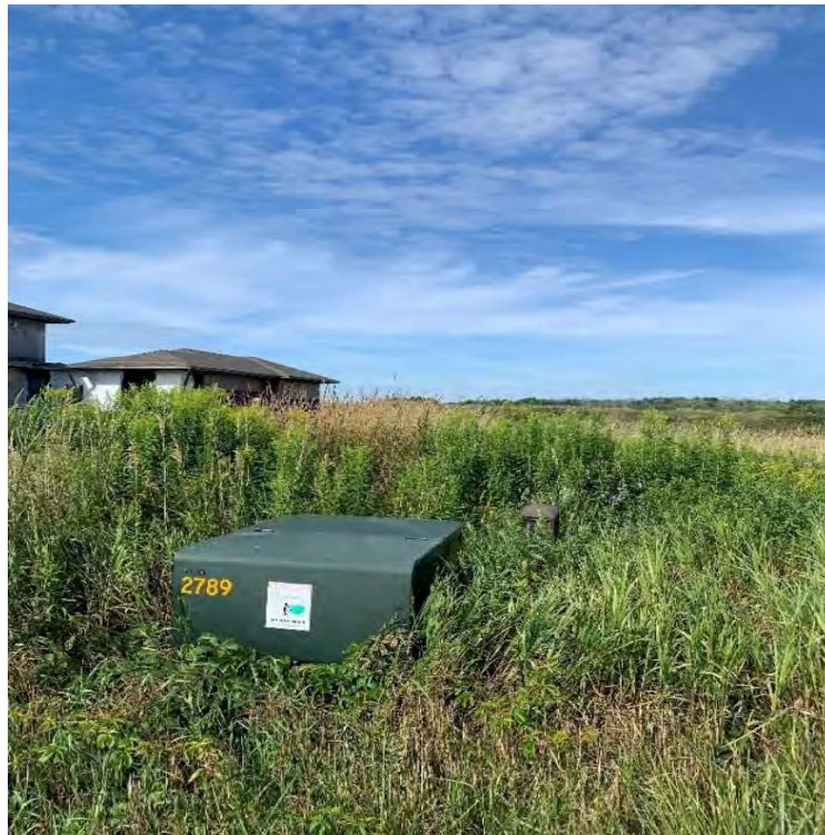
Photo 2: View of pad-mounted transformer along Dale Crescent, facing west.
