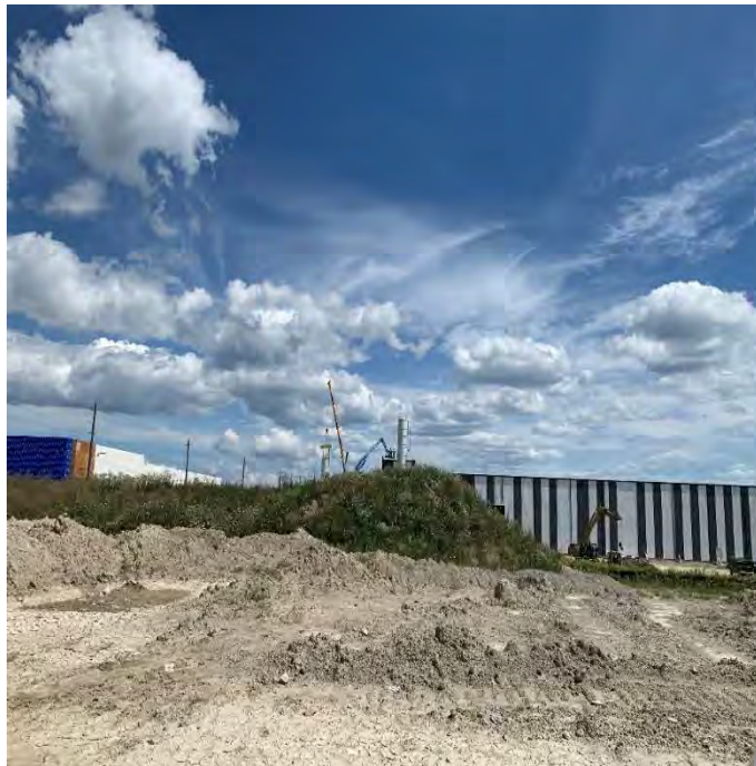
Photo 8: View of fill piles at Site from construction activities along Stirling Crescent, followed by MiTek Canada, facing east.
