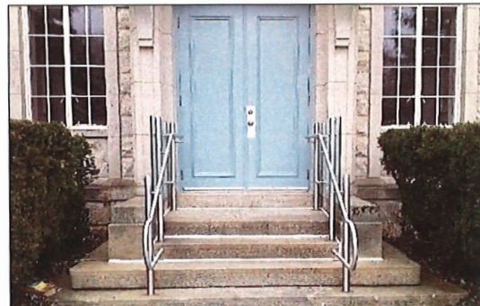
Example of new handrails installed at the main entrance to a heritage building. (Source: GDV)
