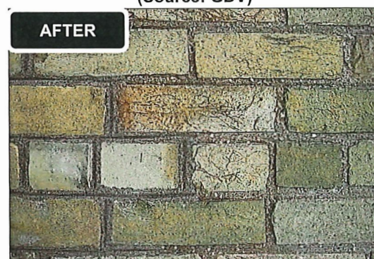
New lime rich mortar is applied to the joints. Repointing work is complete. (Source: GDV)
